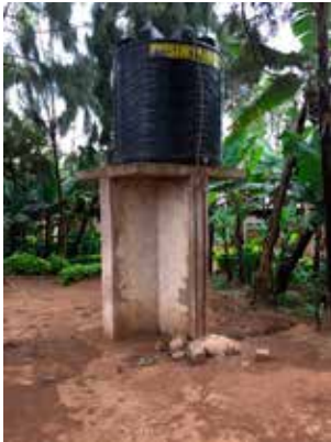
New drinking water tank
